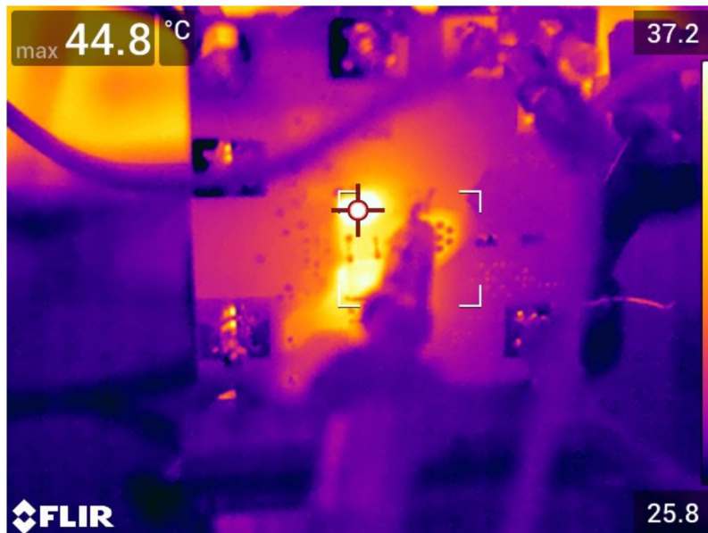
Figure 11 • Thermal imaging with an external fan ( T_{MAX} = 44.8^{\circ}C )
